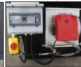
Controls & Primary Burner
